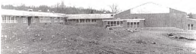
The two above views of the new Penquis Valley High School building show progress being made on the structure which is expected to be open for use next fall. Workmen are finishing rooms on the inside and people in the area are urged to refrain from visiting the construction until such time as it is declared open to visitors. (Staff photos by Mike Brigham)
